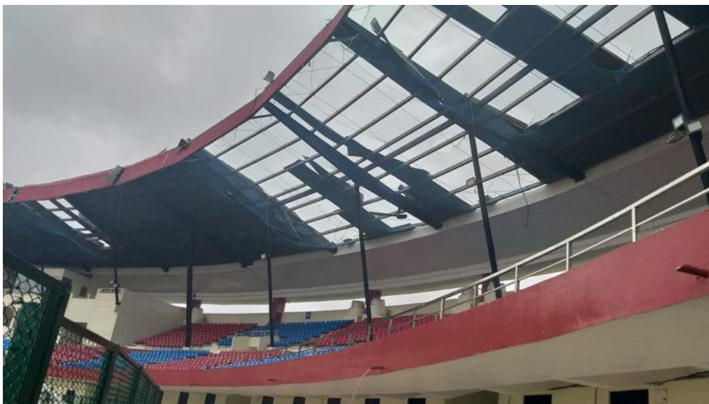
Loss of roof sheeting of Kalinga stadium in Odisha during Cyclone Fani
